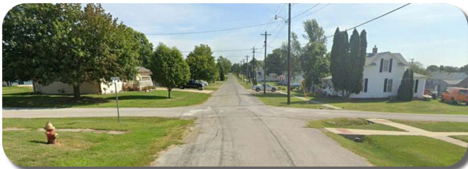
Incomplete sidewalk segments, sidewalks in ill-repair, and lack of ADA accessibility prevent safe pedestrian circulation.
