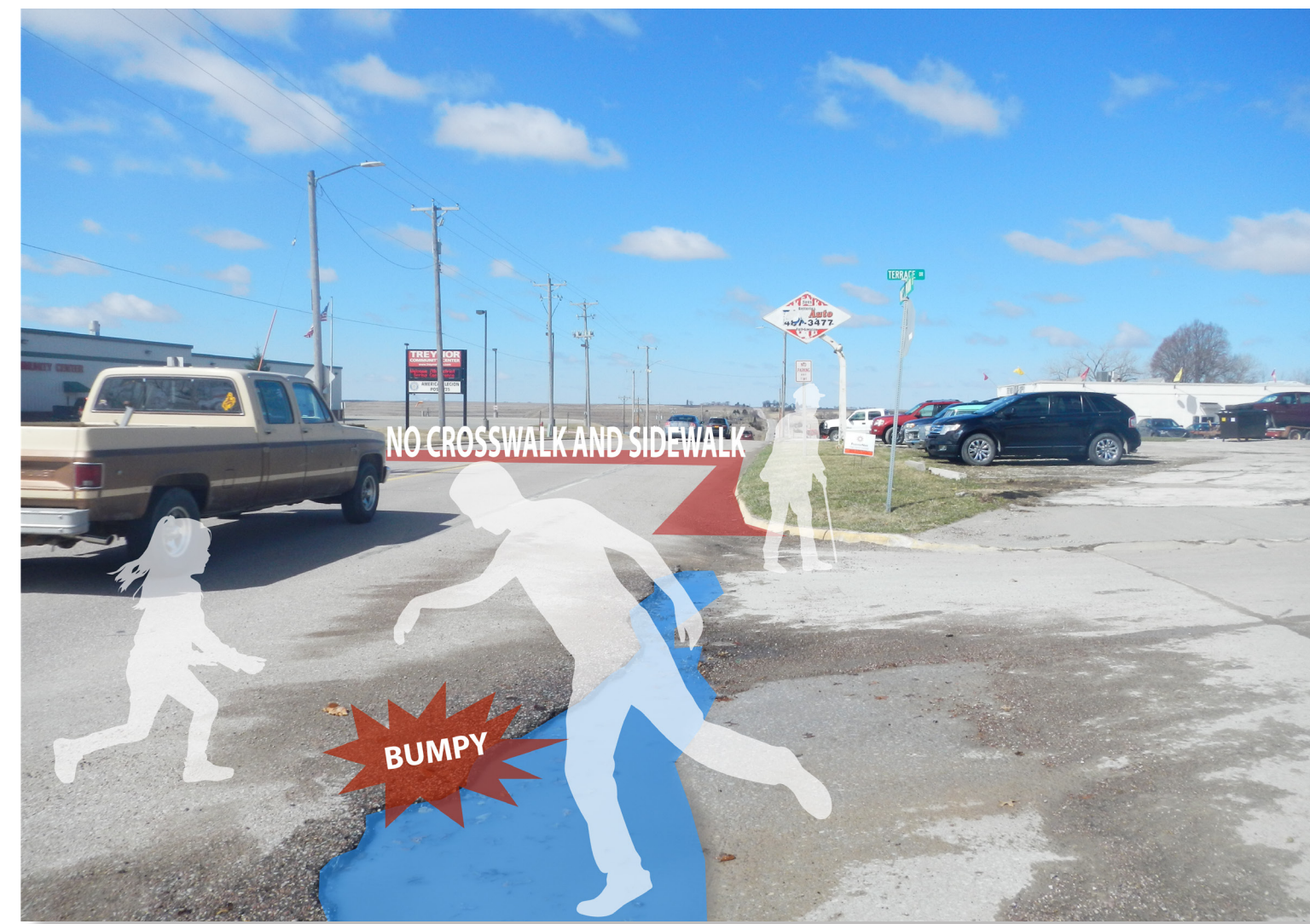
Bumps, potholes and lack of sidewalks along Terrace Rd. limit walking access to Casey's.
