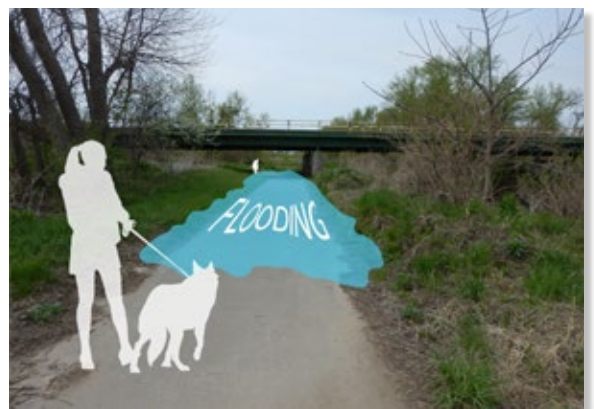
The trail underpass for US Business 30 frequently floods, making it difficult to navigate.
