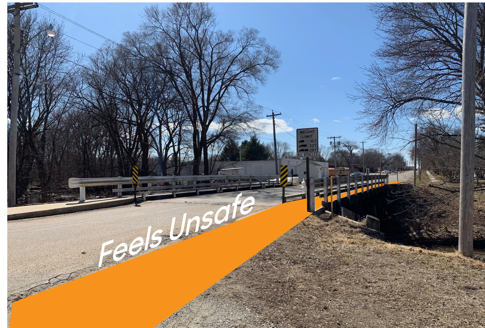
Crossing this bridge feels unsafe, with fast traffic and narrow walkways.
