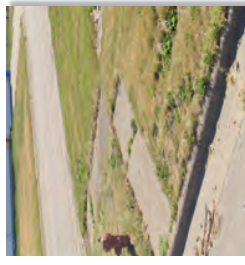
Most of the existing sidewalks in Slater are in poor condition and need improvement.
