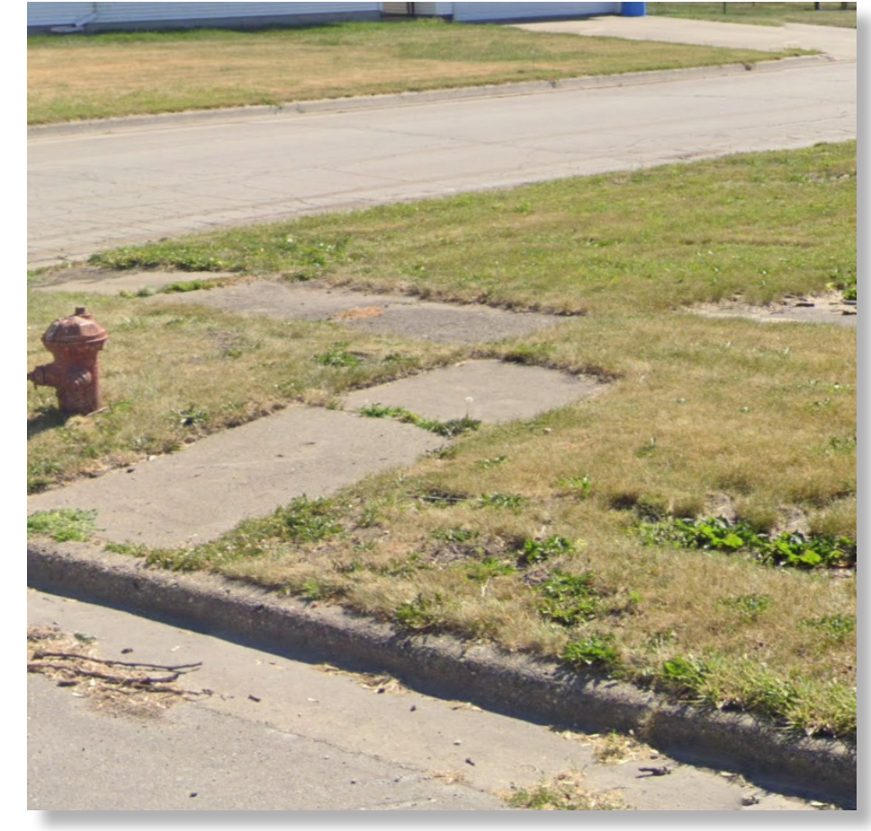
Most of the existing sidewalks in Slater are in poor condition and need improvement.
