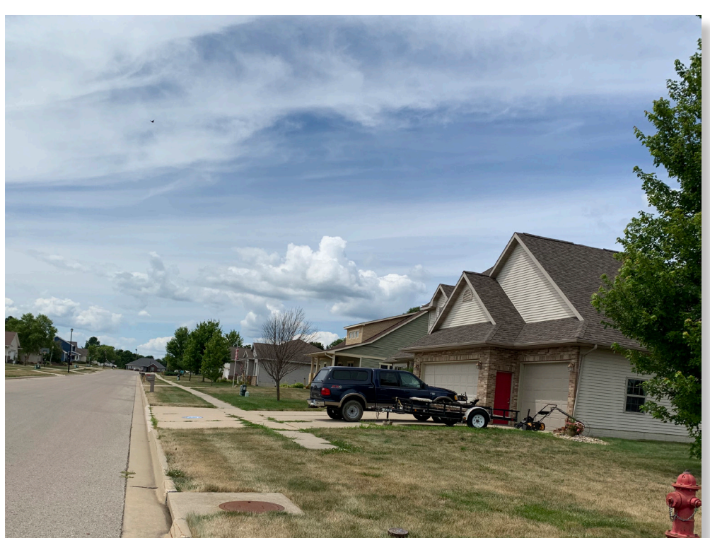
Incomplete sidewalks at Valley Drive
