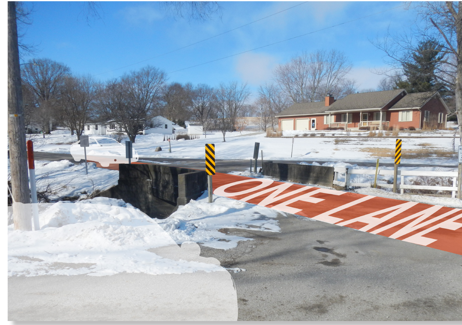
The one-way bridge on West Main Street is aging and creates a bottleneck for transportation into Mingo from the west.
