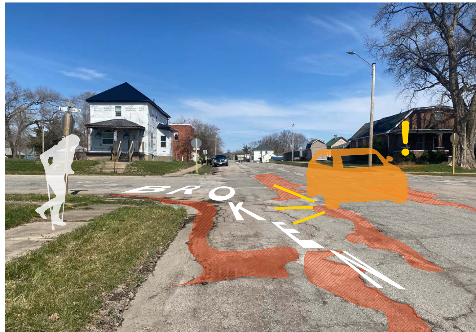
Eighteenth Street is littered with large cracks and potholes that create precarious conditions for drivers and pedestrians crossing the street.
