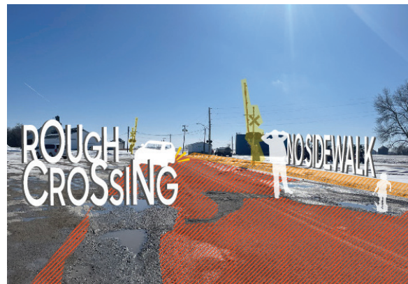
Dips in the roadway and degraded surface conditions make for a rough railroad crossing on Gilmore Street. Pedestrians do not have dedicated access along this route or for crossing the tracks.
