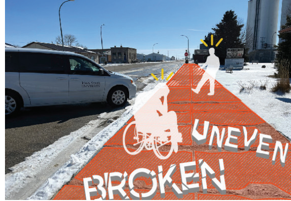
Old, broken, and uneven sidewalks along Gilmore Street impede access for many users in the downtown.
