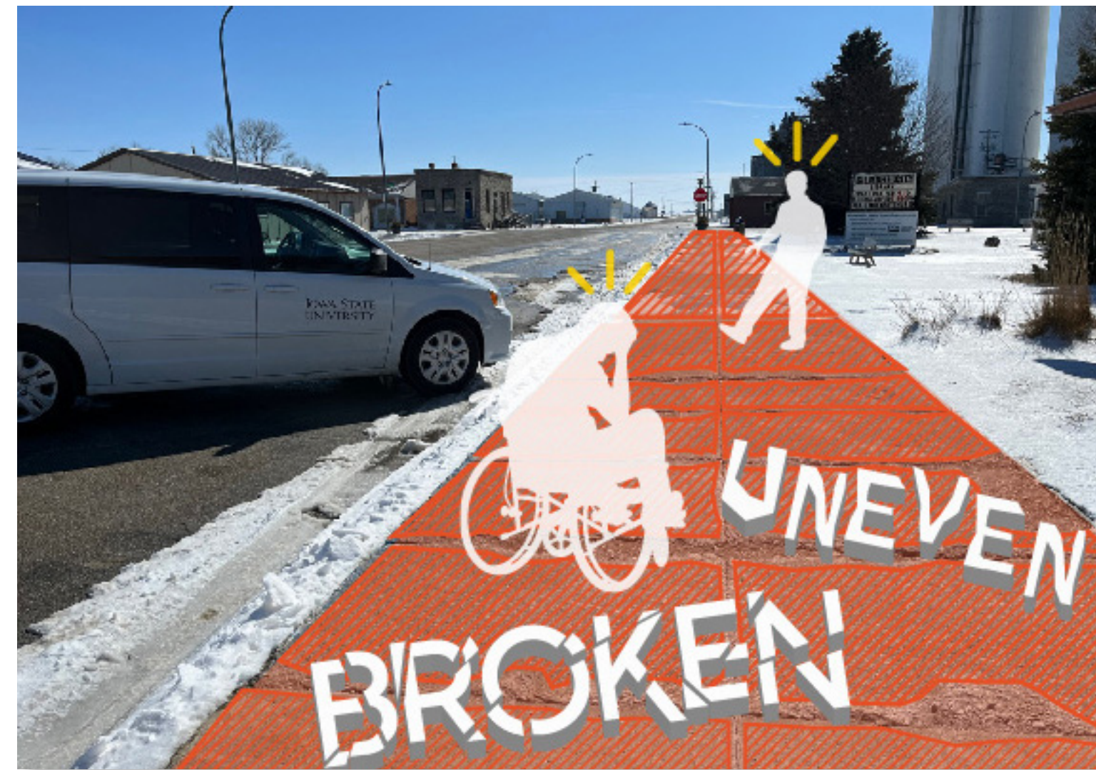
Old, broken, and uneven sidewalks along Gilmore Street impede access for many users in the downtown.
