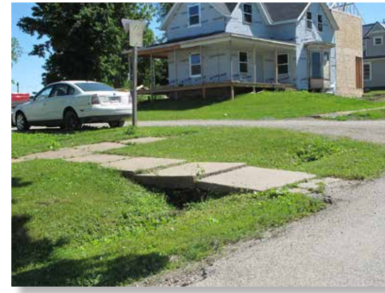
Existing conditions: Structural issues.
