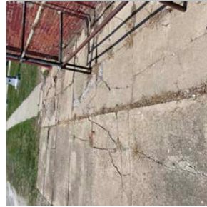
Most of the existing sidewalks in Farragut are deteriorating and need improvement.
