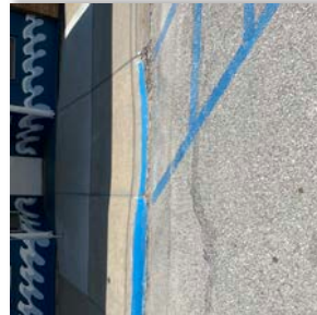
A ramp in downtown is not up to current ADA standards for those with mobility limitations.
