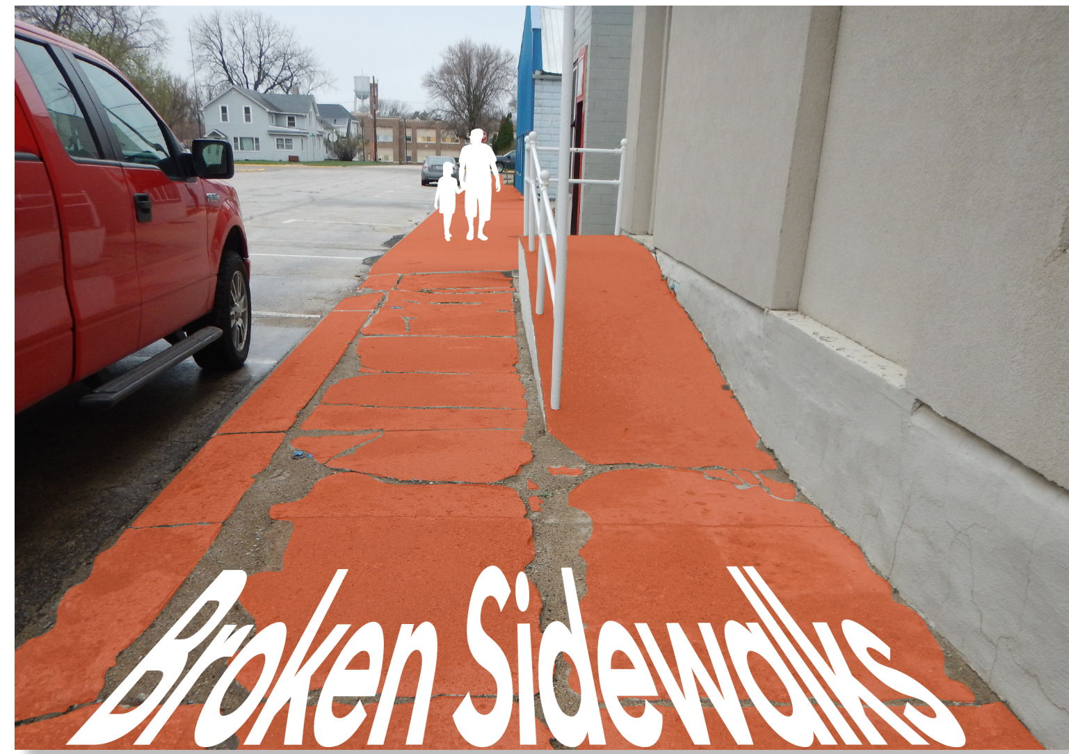
The broken sidewalks along 10th Street are just one example of poor sidewalks in Emmetsburg.
