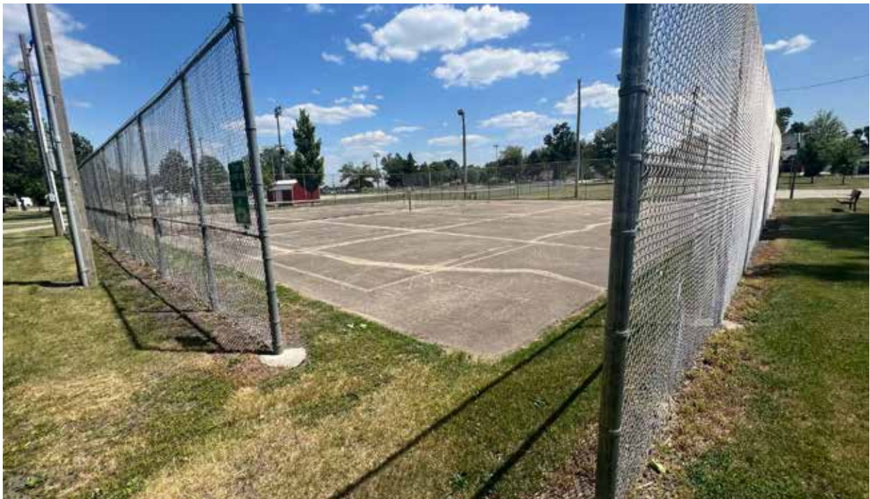
Existing tennis courts to be resurfaced for one pickleball court and one tennis court
