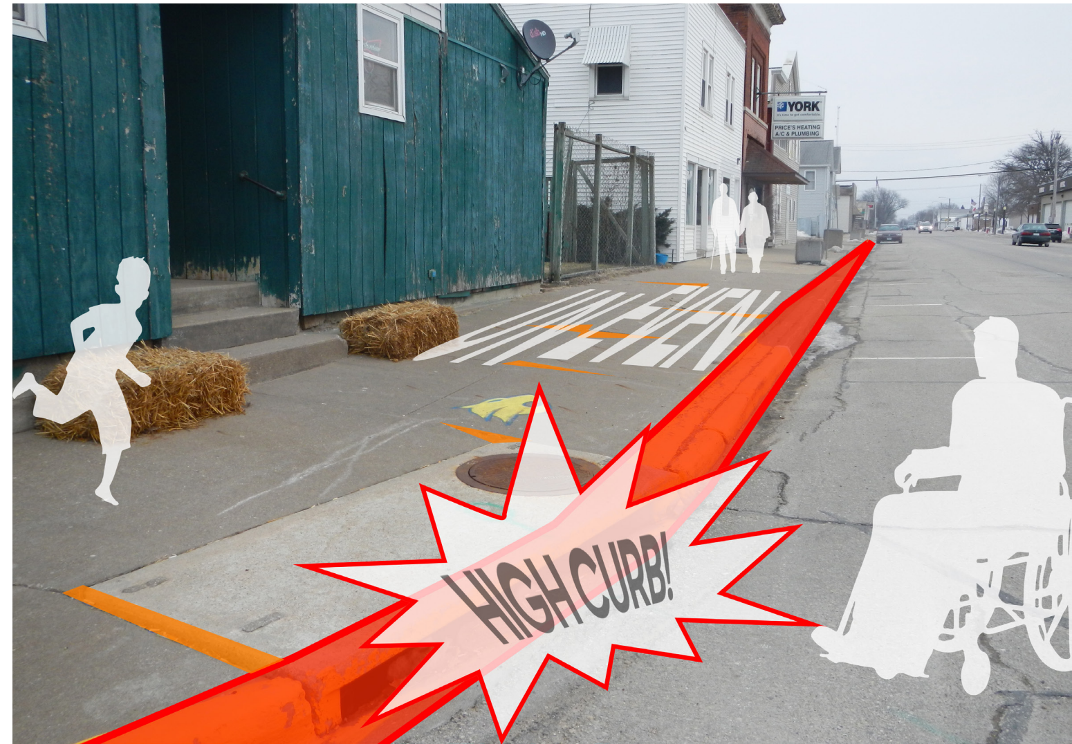
The sidewalks on Main Street are uneven and are difficult to access from the street because of the two-step curb, especially with snow in the winter.
