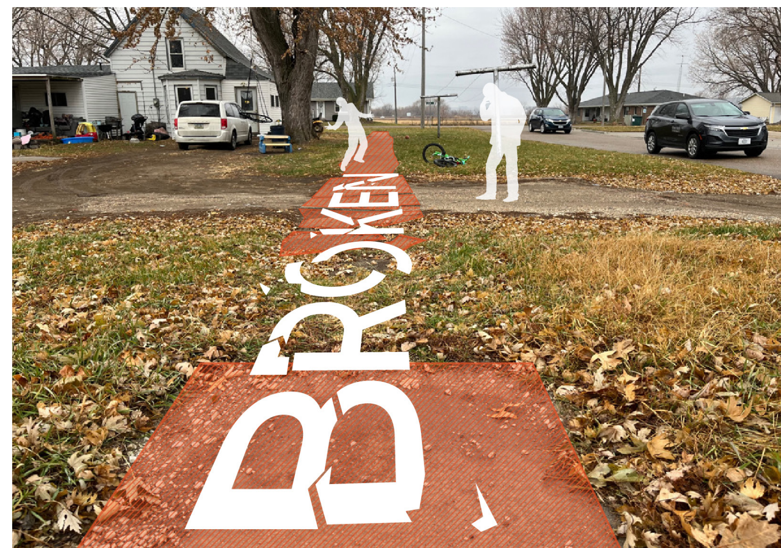
Myrtle Street's sidewalks are heavily worn and incomplete, forcing people to walk in the roadway.
