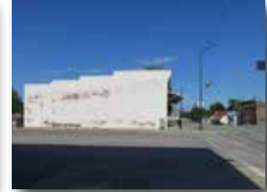
City Library: Facade Maintenance Req.
