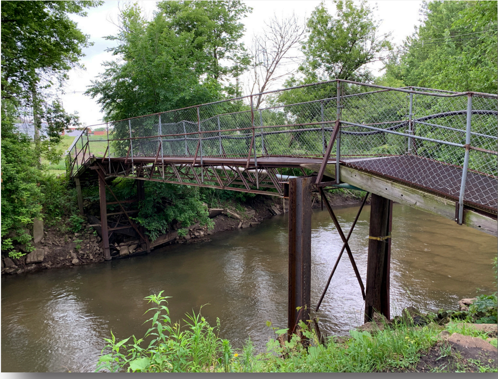
Pedestrian Bridge at Savage Park: Not ADA compliant
