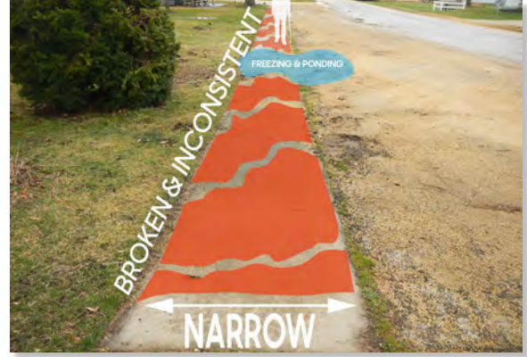
The sidewalks along 2nd Street are narrow, broken, and inconsistent causing residents to walk in the street.
