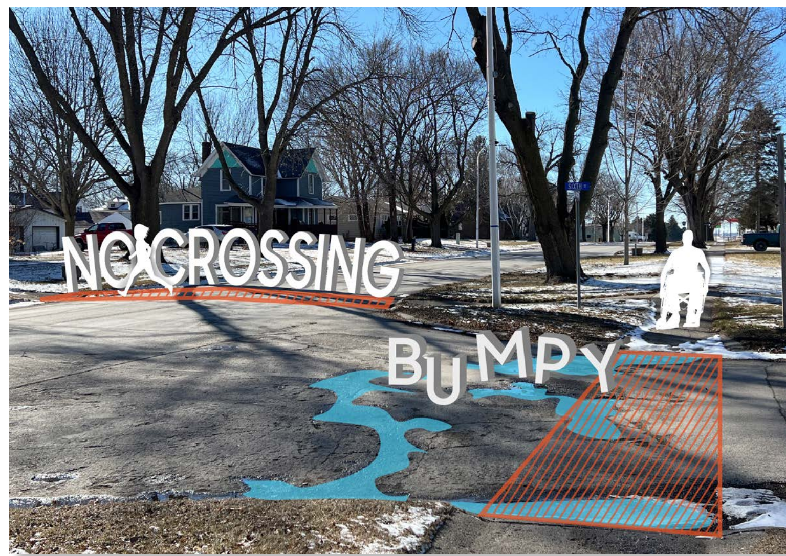
Walnut Street sidewalk conditions make traversing intersections difficult for pedestrians and cyclists.
