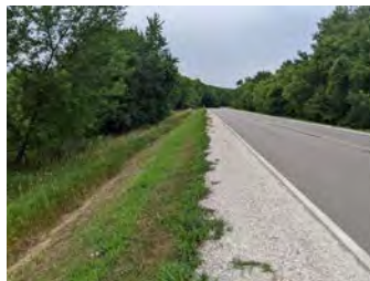
5 Steep ditches along Orton Road
