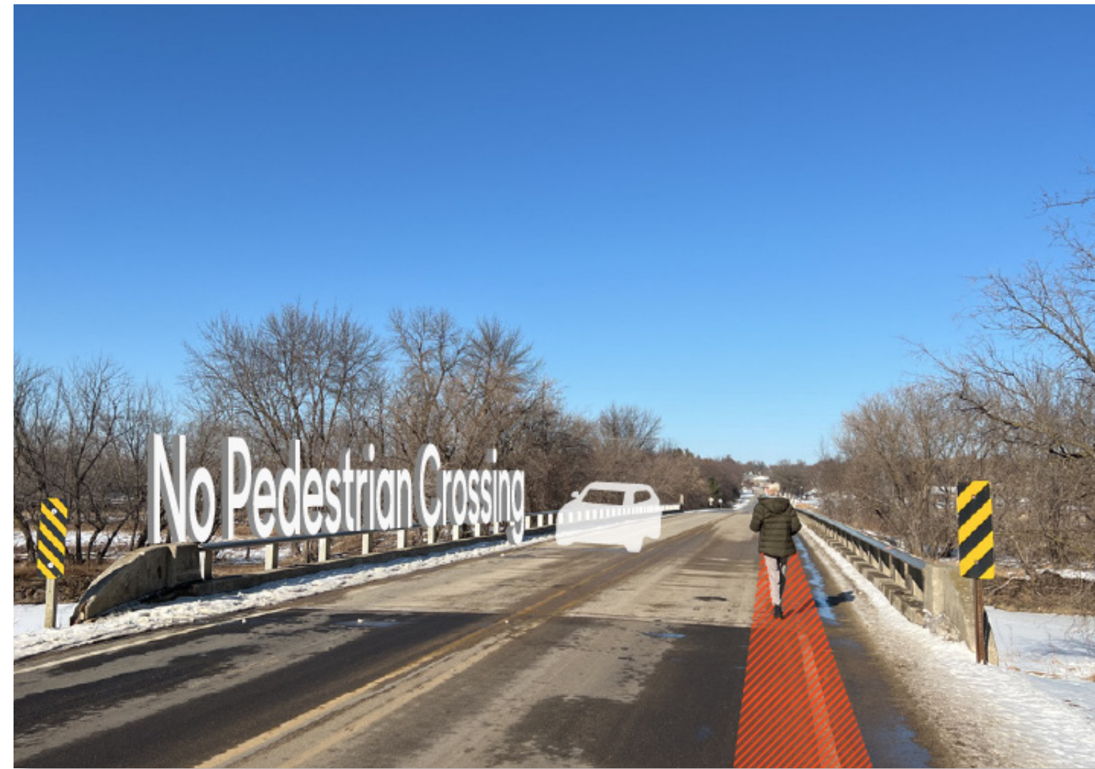
Lack of sidewalks at the bridge over the river on Orton Road creates a disconnect between town and the neighborhood and park to the southwest.
